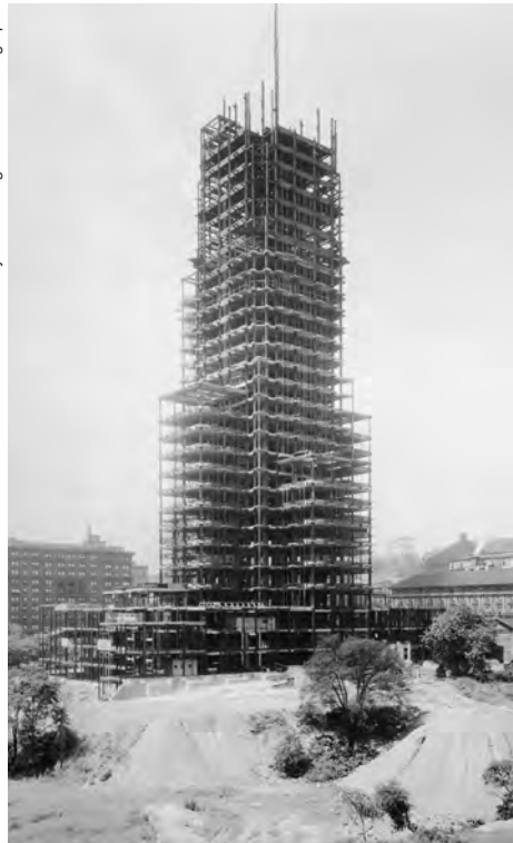
Construction, which began in 1926, persisted throughout the 1930s, despite the Great Depression.
