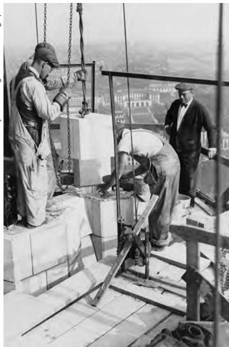
Workmen install blocks of Indiana limestone on the top floors of the tower.
